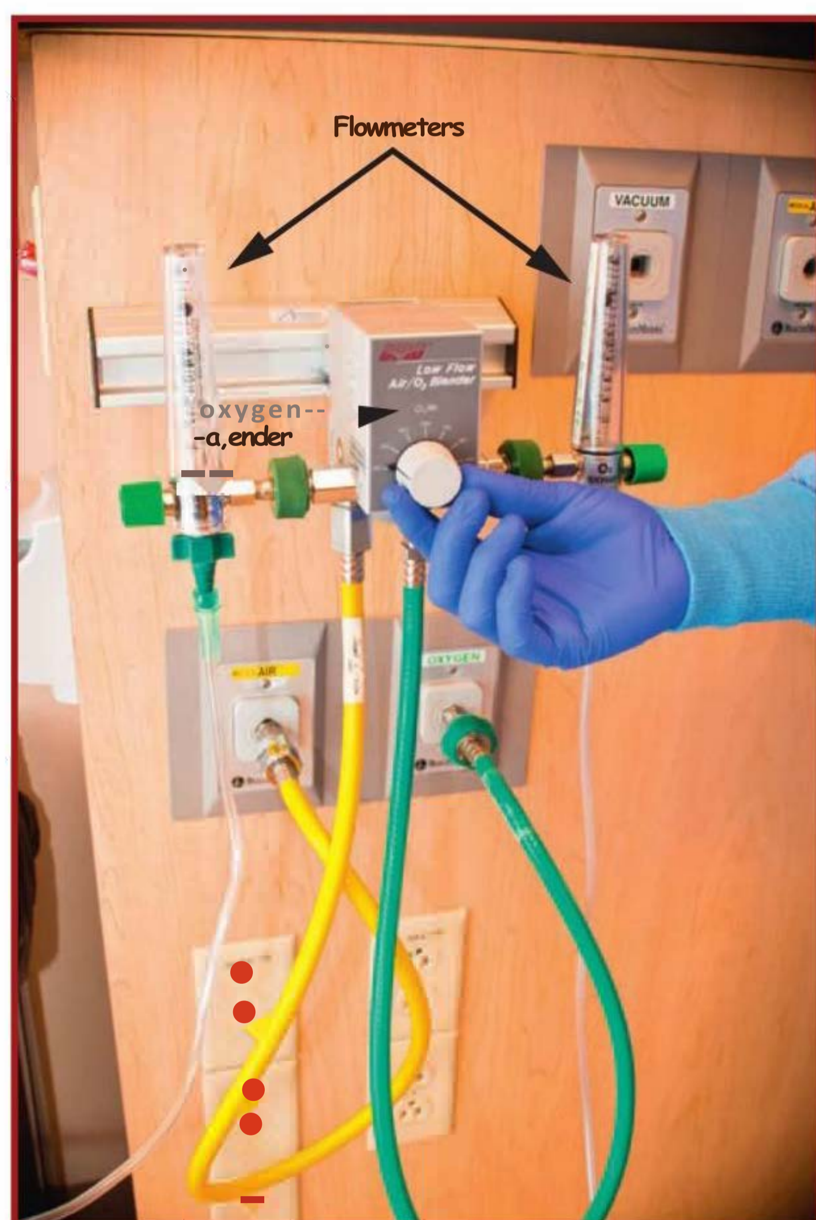
Figure 3.17. Adjust the concentration and flow of oxygen with compressed air (inflow from yellow hose), compressed oxygen (inflow from green hose), an oxygen blender, and a flowmeter. The image shows 2 flowmeters attached to the oxygen blender. Your system may only have 1 flowmeter.
